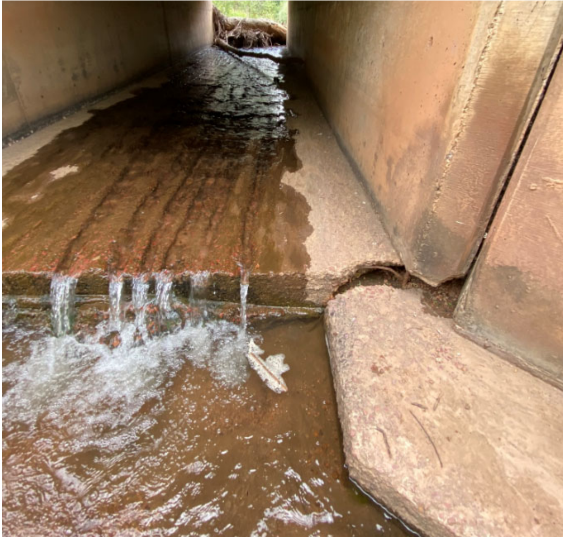
Picture 2 – Exposed Footing, Erosion, Wingwall Separation
